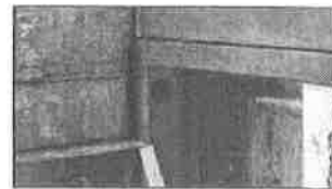
PHOTOGRAPHS ABOVE AND ABOVE RIGHT SHOWING SOUND PROOFING ELEMENTS ON SITE WHICH STOP THE SOUND PROOF WALL FROM TOUCHING THE EXISTING STRUCTURAL WALL
